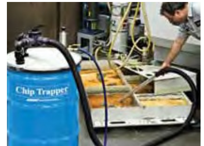
Chips can accumulate in the sump, restricting coolant flow.
